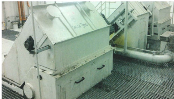
Discharge End of a VacuFilter E-Series Central Coolant System, supplied to a steering component manufacturer
